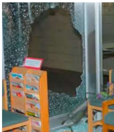
The broken window
